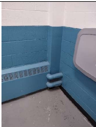
Women's Room radiant baseboard.
