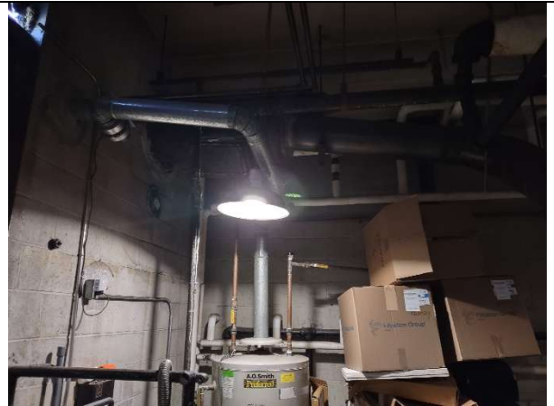
Limited traditional lighting in the boiler room.
