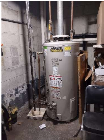
Natural gas fired hot water heater.
