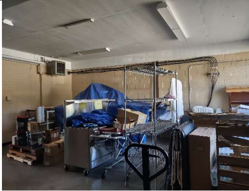
Unit heater in storage room
