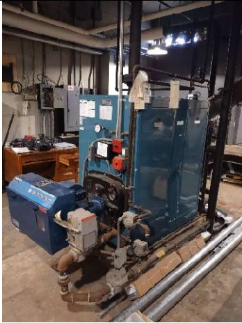
Natural gas fired 1260 MBH burner and boiler.
