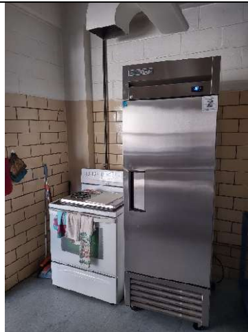
Ductwork in kitchen to be reworked to match new stove with ceiling plan.
