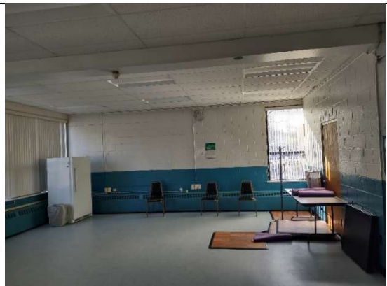
Corner meeting room radiant baseboard.
