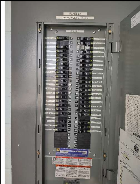
225 amp 120/208 volt lighting panelboard, installed 2018
