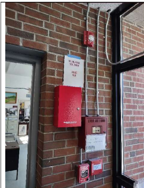
The main fire alarm panel. There were no violation notes on the front cover.
