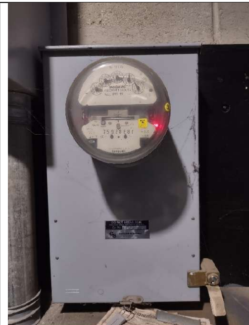
Meter for electrical service.
