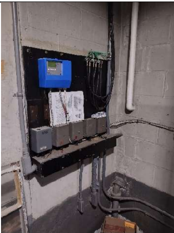
More recently installed temperature controls.
