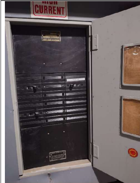
Sub panel original to the facility.
