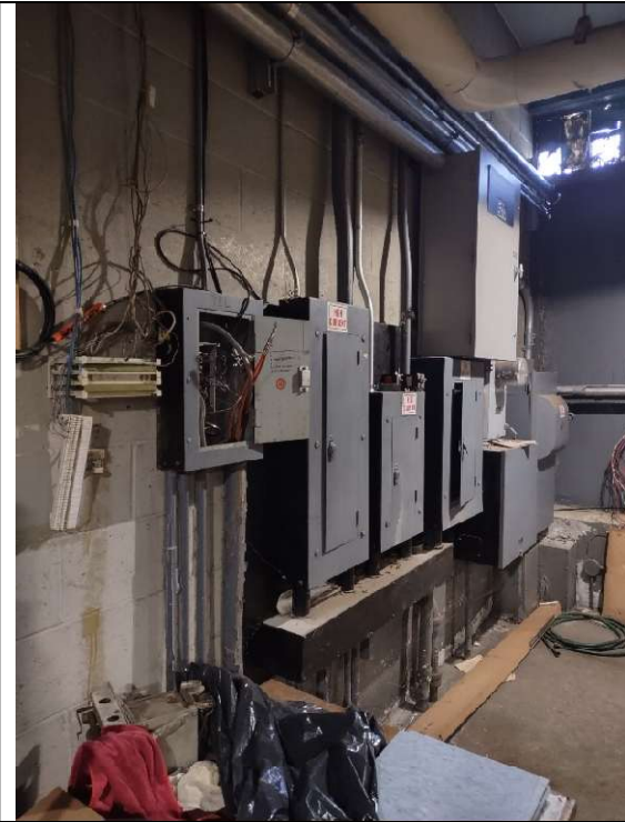
The main service equipment is in the basement. Functional but past its service life.
