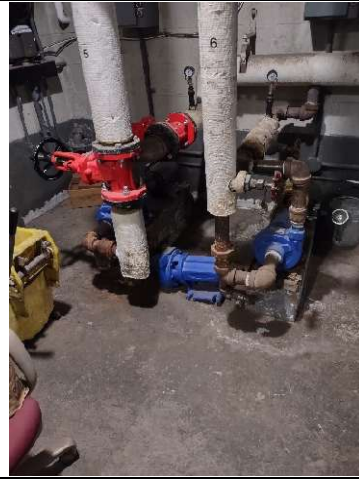
Hot water circulation pumps and spare.
