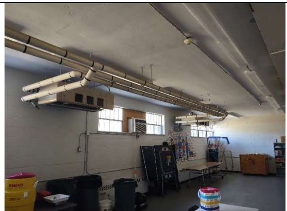
AHUs, radiant baseboard, and t-stat in the storage room.
