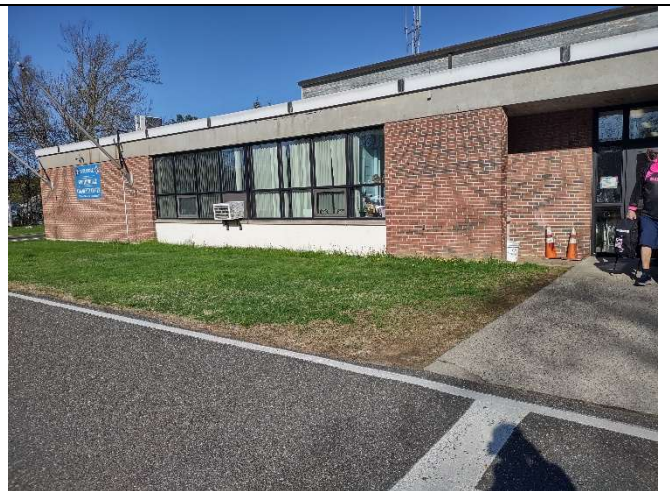
Exterior flood lights with LED bulbs but showing signs of age.
