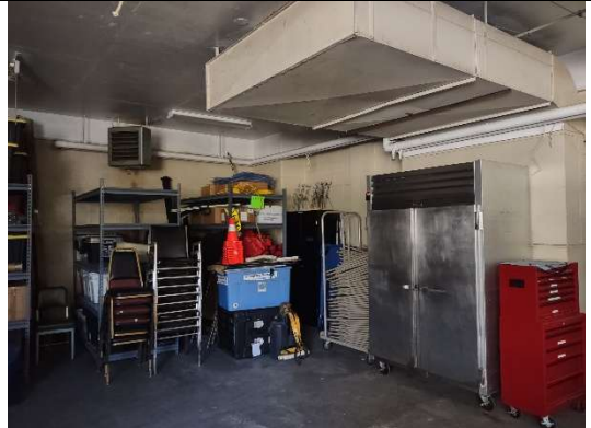
Unit heater and exhaust ductwork.
