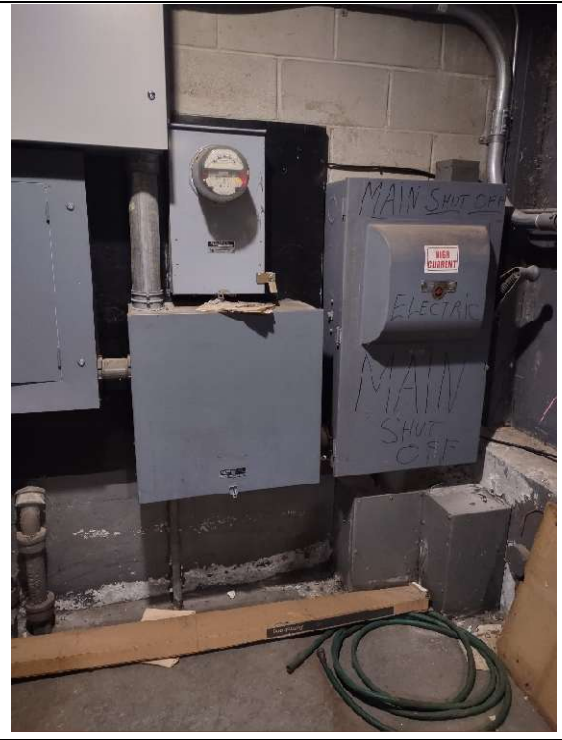
400 amp, 240 volt, three phase service disconnect switch. This is fed directly from the pole mounted transformer. Note the overall condition shows that equipment is past its expected service life.
