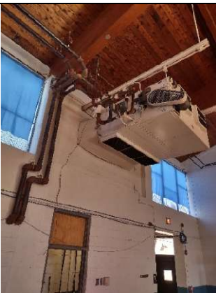
The single working AHU in the gym
